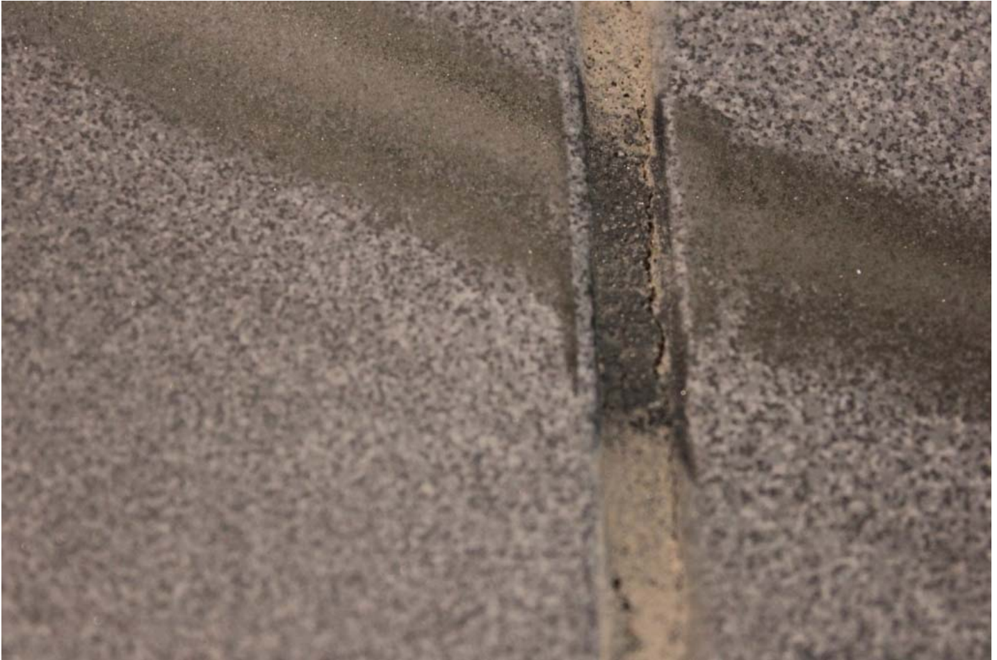
Image 2: Cracked grout joint
